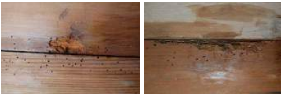
Wood worm damage on back of panel
