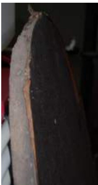
Damage to top of frame
